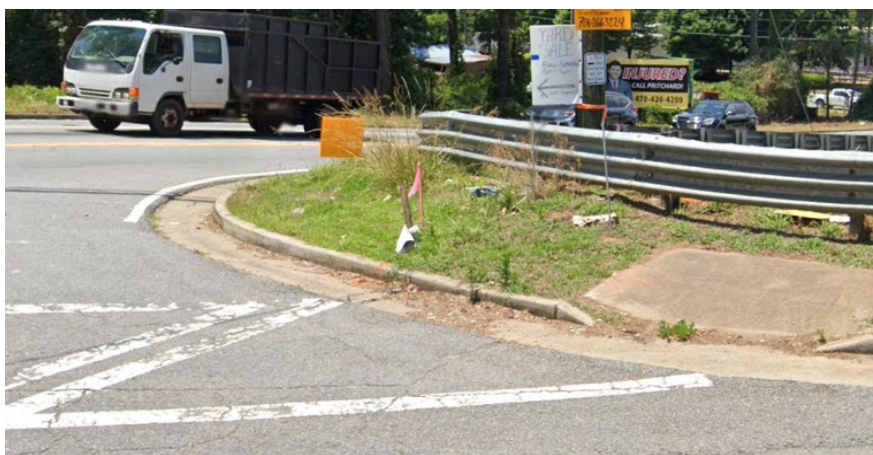
Missing sidewalk connection on northwest corner of intersection
