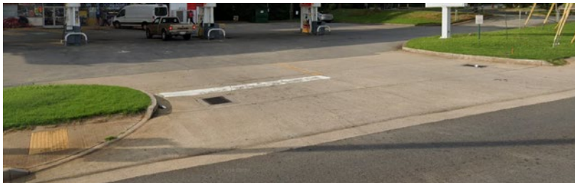
The north-leg of the intersection is missing a marked crosswalk
