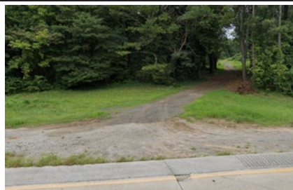
Northbound looking west. A maintenance turn-around is missing signage
