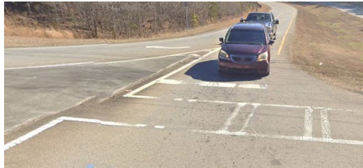
Many intersection markings have faded
